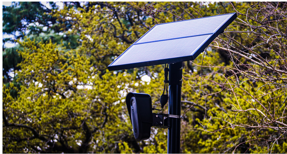
Photo by Alyus Dick Flock camera located on Hebrard Blvd.
